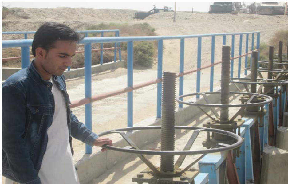
Figure 4; Regulator over Lashkari Canal for controlling flow of water during different seasons
