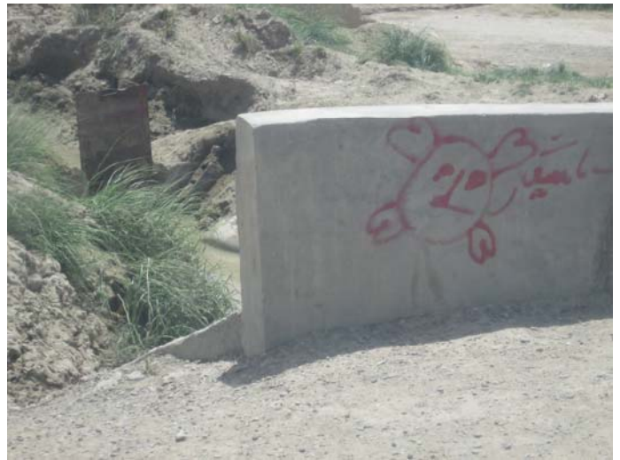
Figure 23; Sub-canal of Haji Yaseen, Jui Amnient Mali irrigates 60 hectare area
