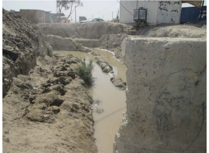
Figure 25; Sub-canal of Haji Taher Arab gets water from Lashkari Canal irrigates 100 hectare area
